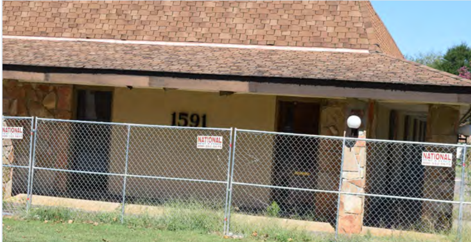
Building 1591 - Burned / Down Unit
