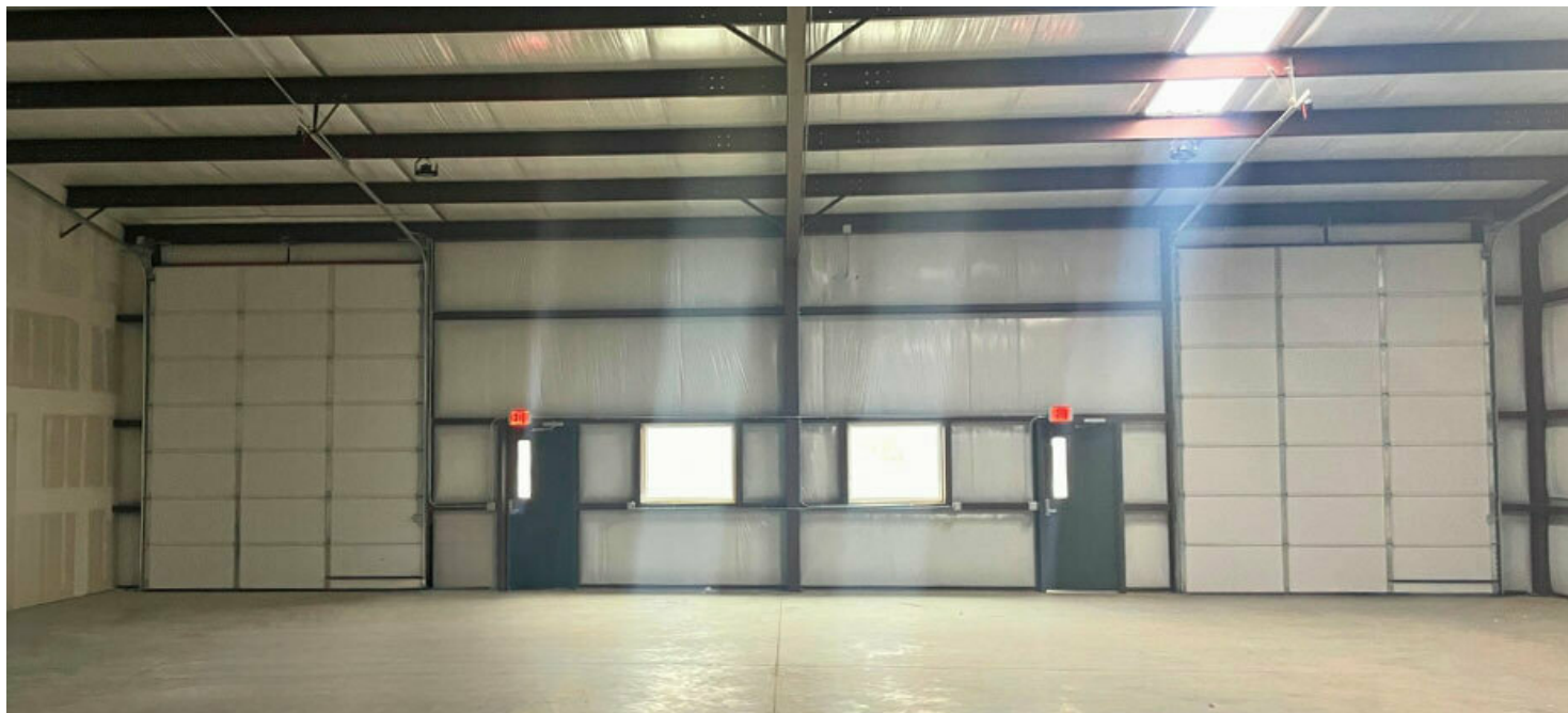
Front Overhead Doors
