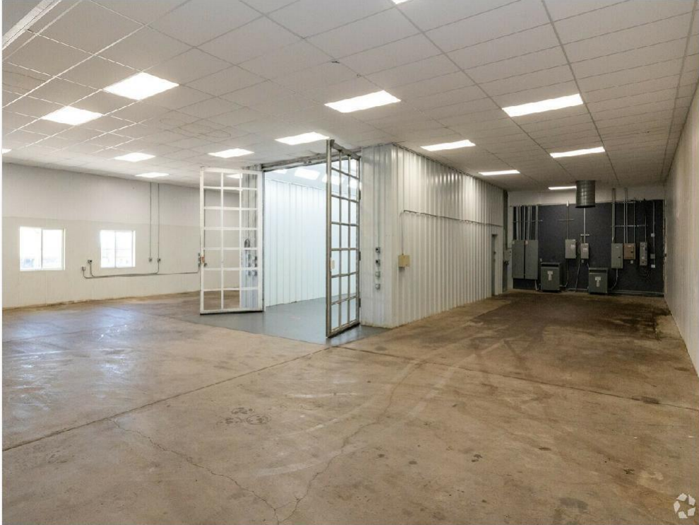
PAINT BOOTH AND ELECTRICAL SERVICES
