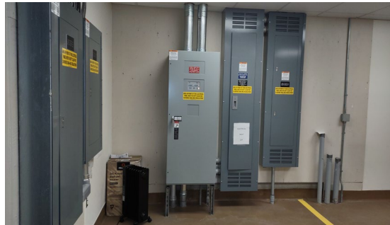
1 st Floor Electric w/automatic transfer switch
