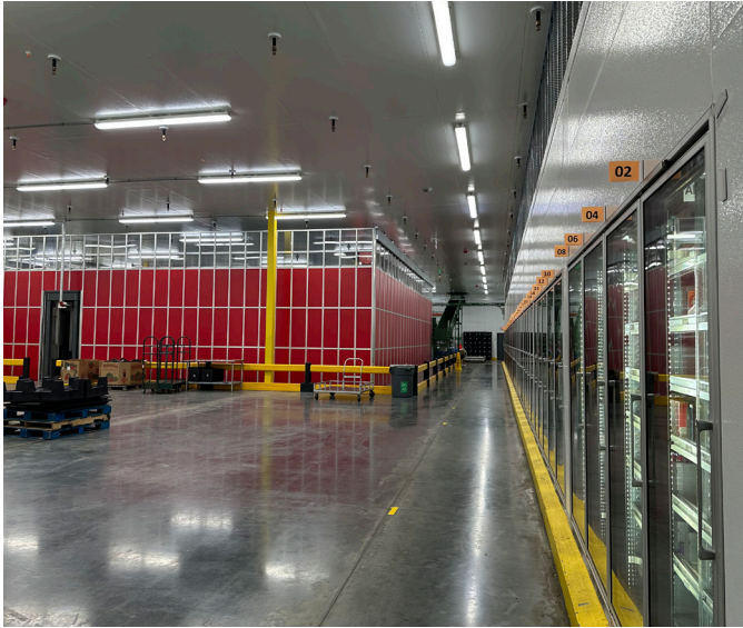
Cooler / Automated Pick Area
